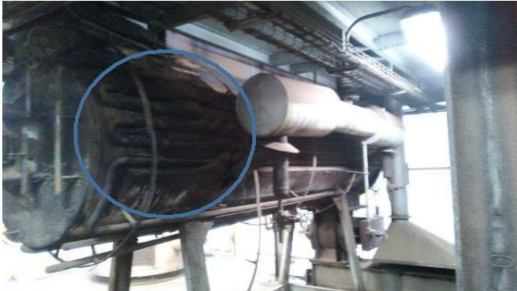
Figure 3.56 Shows totally damages of pop cork chamber in GMT section 1
