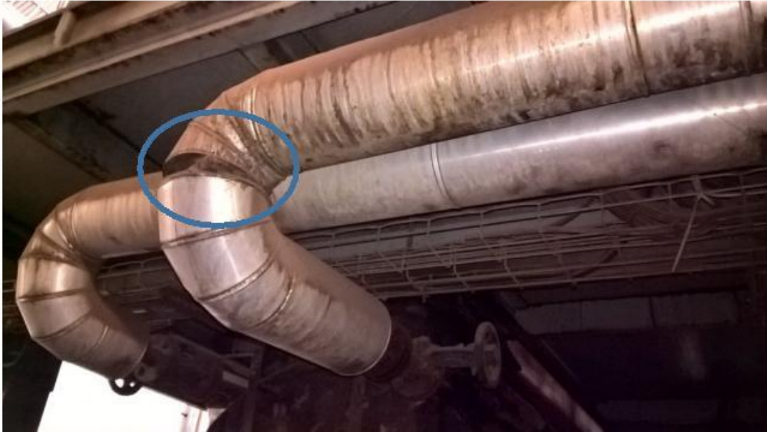
Figure 3.58 Show detail views of dislocation of pipes in pop cork chamber present in GMT section 1
