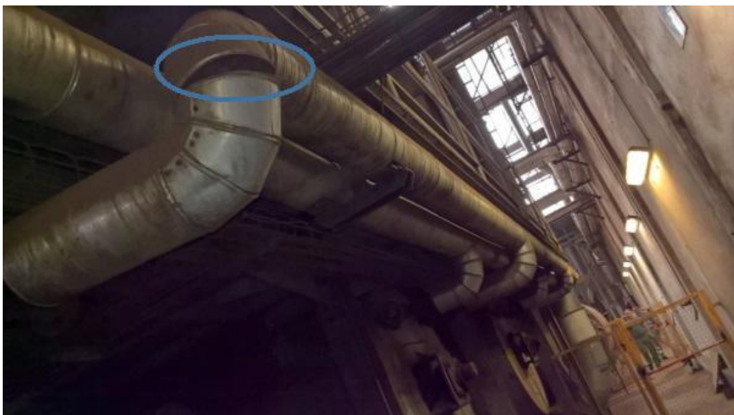
Figure 3.57 Shows breakages in the pipe lines of cork passing in pop cork chambers
