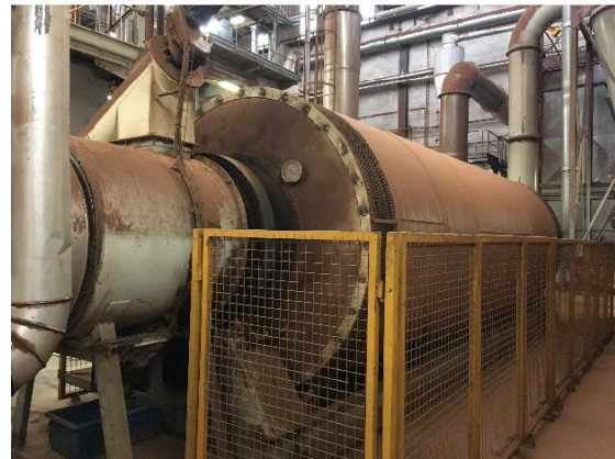
Figure 3.24 Dryer in GMT section 3
