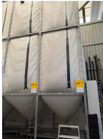
Figura 4 - Silos de EPS.
