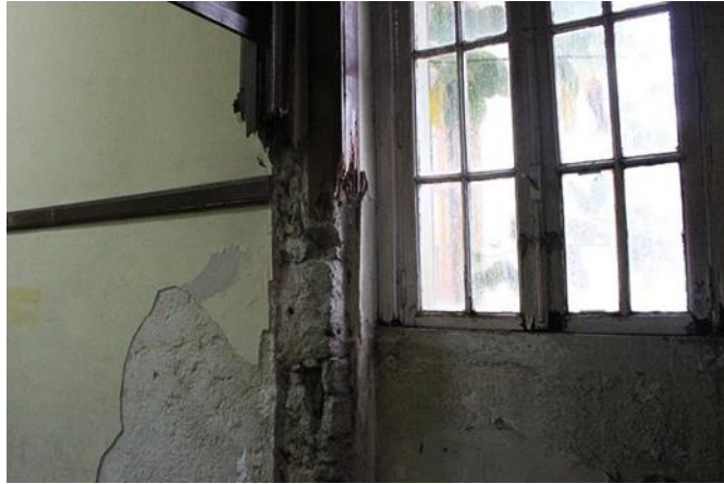
Figure 21-Signs of Degradation in the walls
