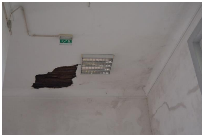
Figures 22 and 23- Signs of Degradation in the Ceiling
