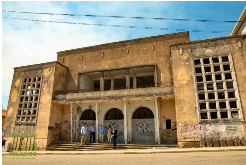
Figure 41 -The condition of the building when acquired by the Municipality
