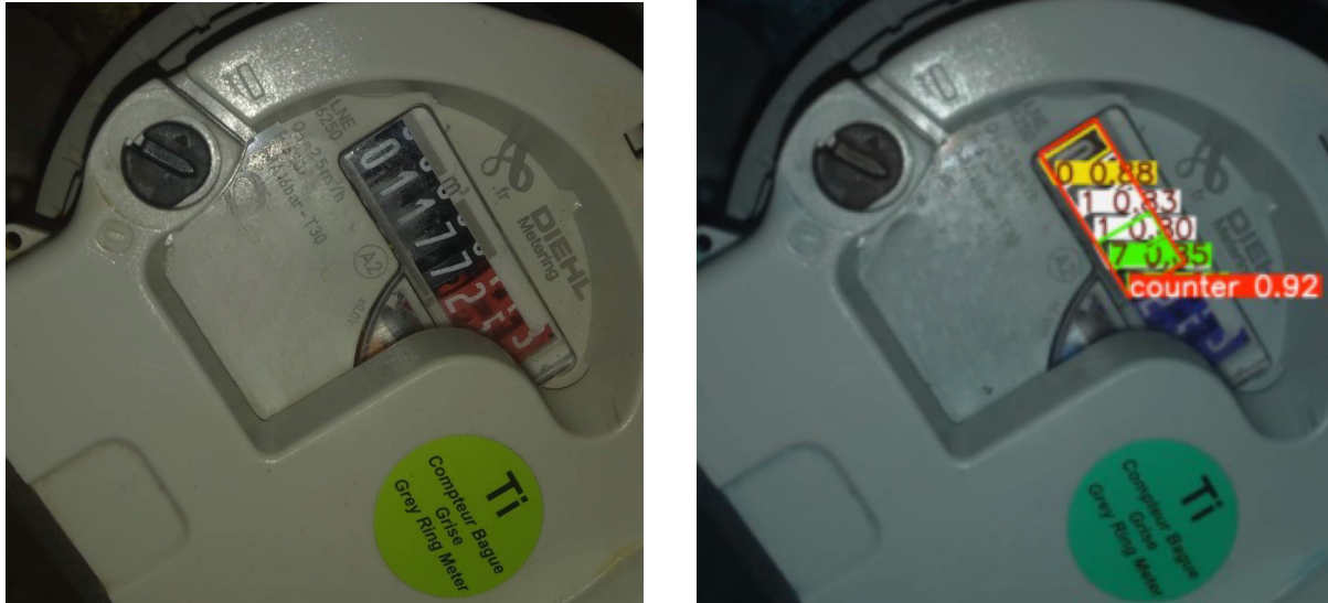
(a) Water Meter
