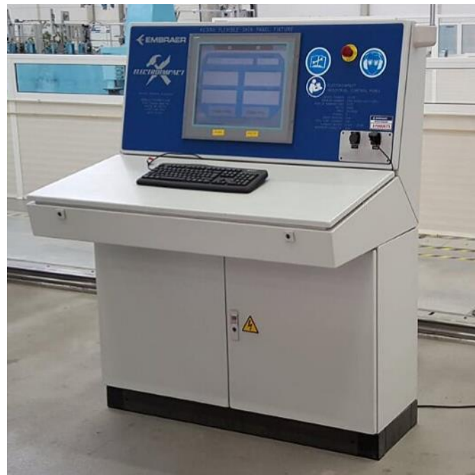
Figure 13 - Flex Fixture main controller
