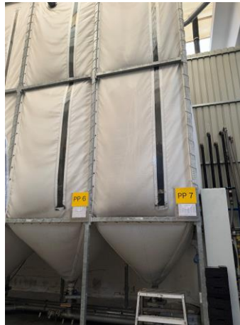
Figura 4 - Silos de EPS.
