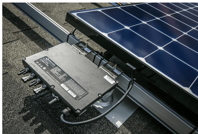
Figure 13– Microinverter installed next to the photovoltaic module [48]
