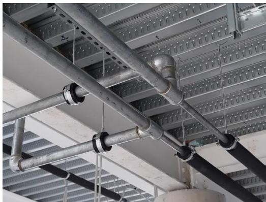
Figura 38 – Circuito Chilled Water e Heating instalado PCC.
