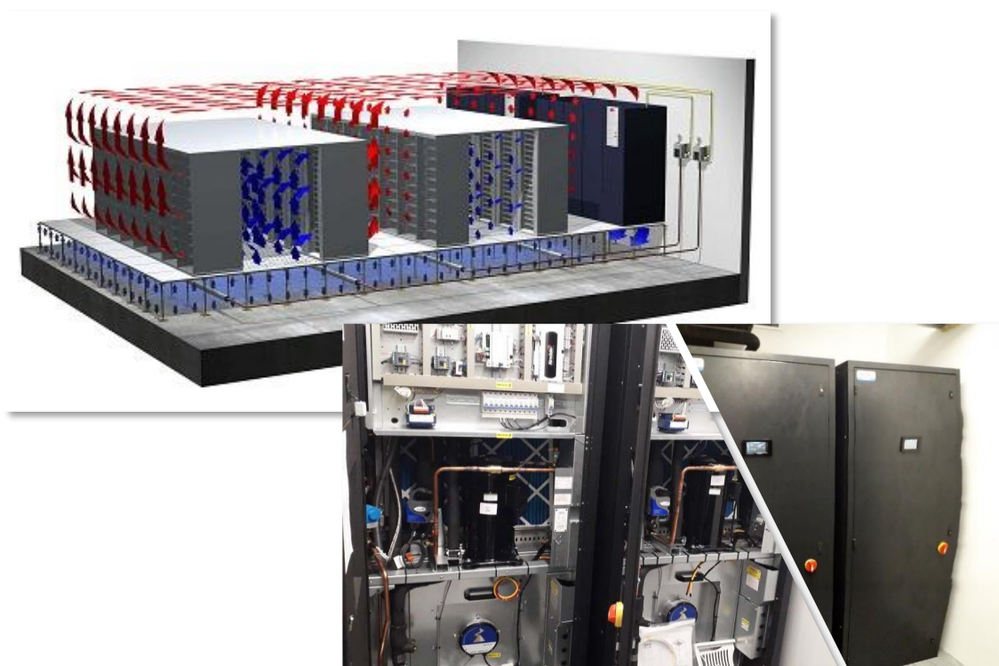
Figura 33 – Sistema Close Control instalado no CPCC (AthenaAir)
