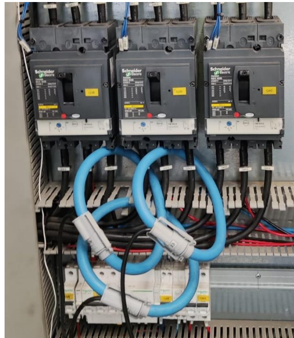
Figure 55 Addition of current transformers for monitoring the second loop feed section.
