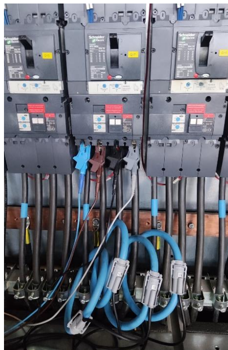
Figure 35 Introduction of monitoring equipment at the stacker crane feed point.
