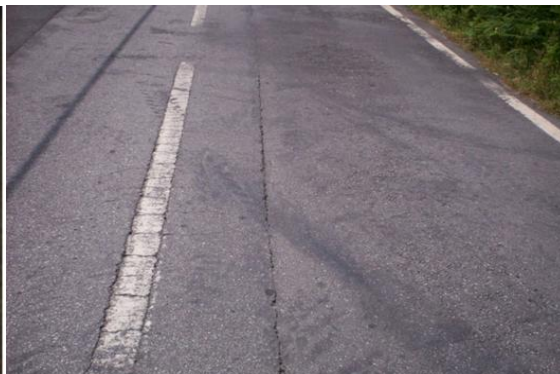
Figura 21 – Fenda Longitudinal Lateral (Jacob, 2013)
