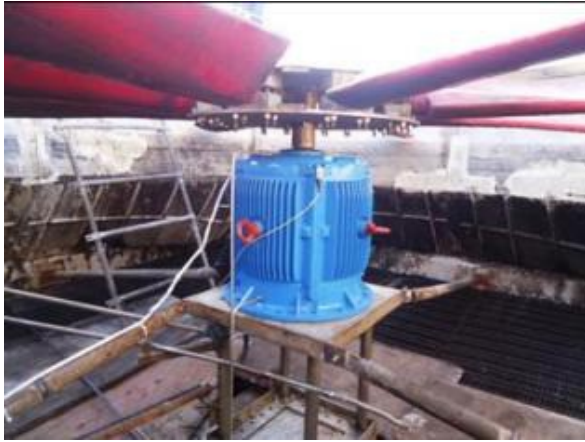
Figure 10. Cooling tower with PM motor
