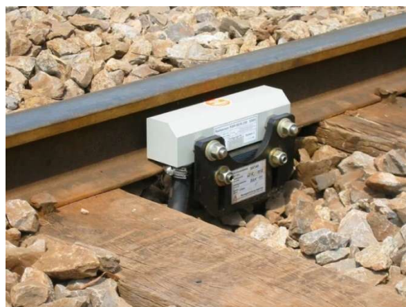
Figure 2.6: Axle counter installation on the track. (Argenia, s.d.)
