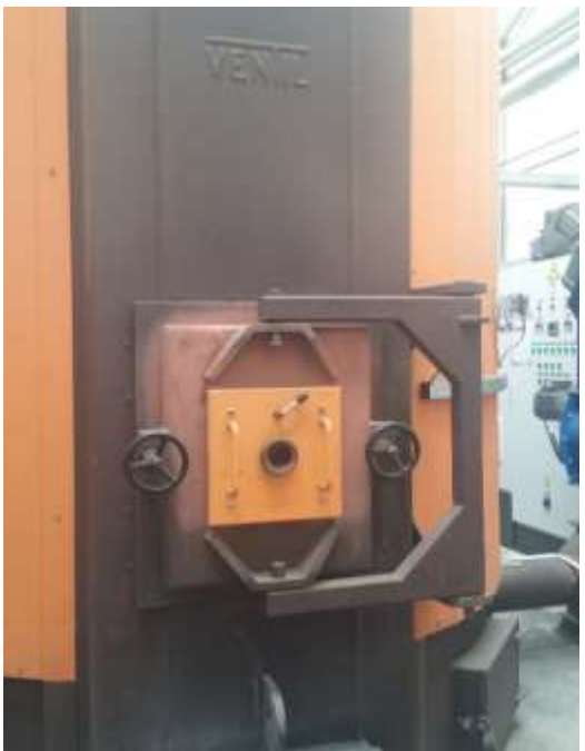
Biomass Manual Inlet
