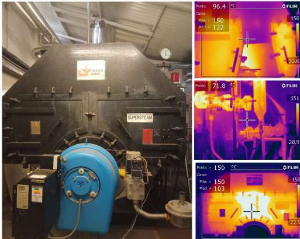
Figure 6.5.1 – Steam generator and thermal pictures
