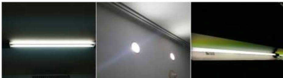
Figure 6.3.1 - Existing lighting system
