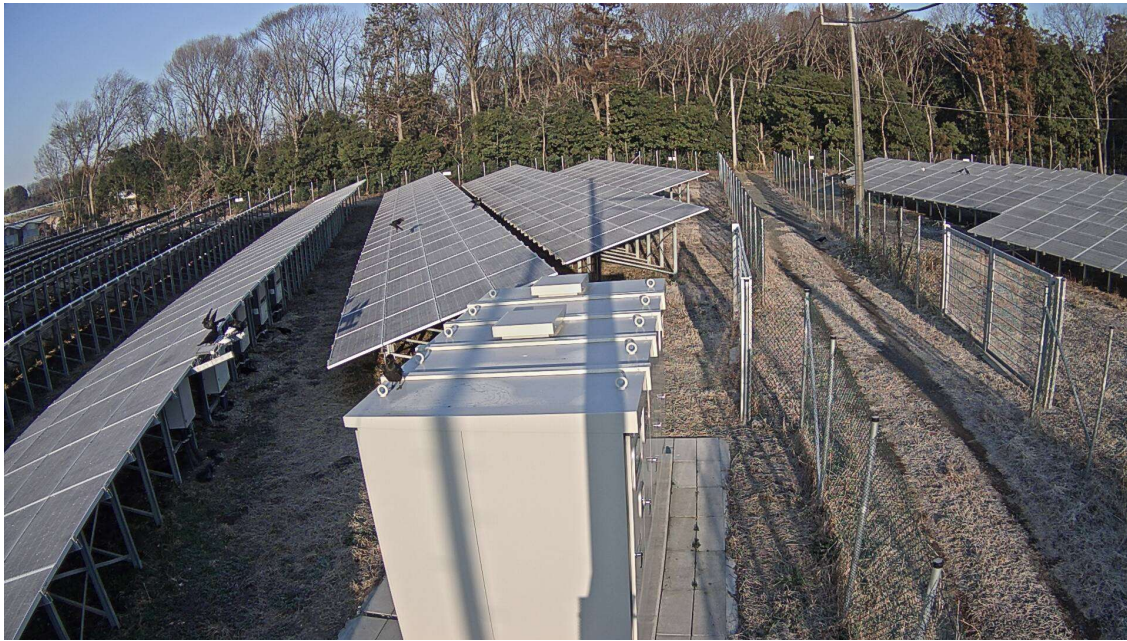
Figure 55 - Birds resting on the irradiance sensors and modules during winter.
