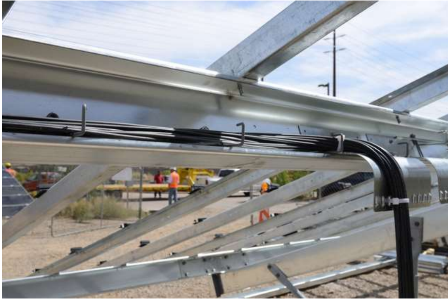
Figure 43 - String cables running inside the MMS.
