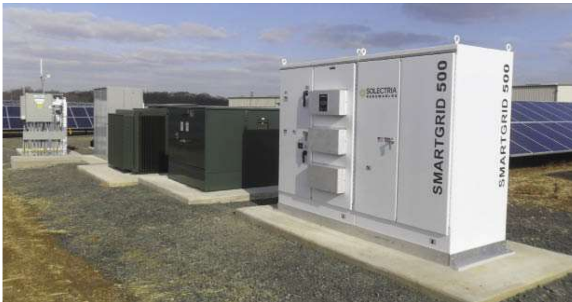
Figure 28 - Transformer station next to Smartgrid central inverters.
