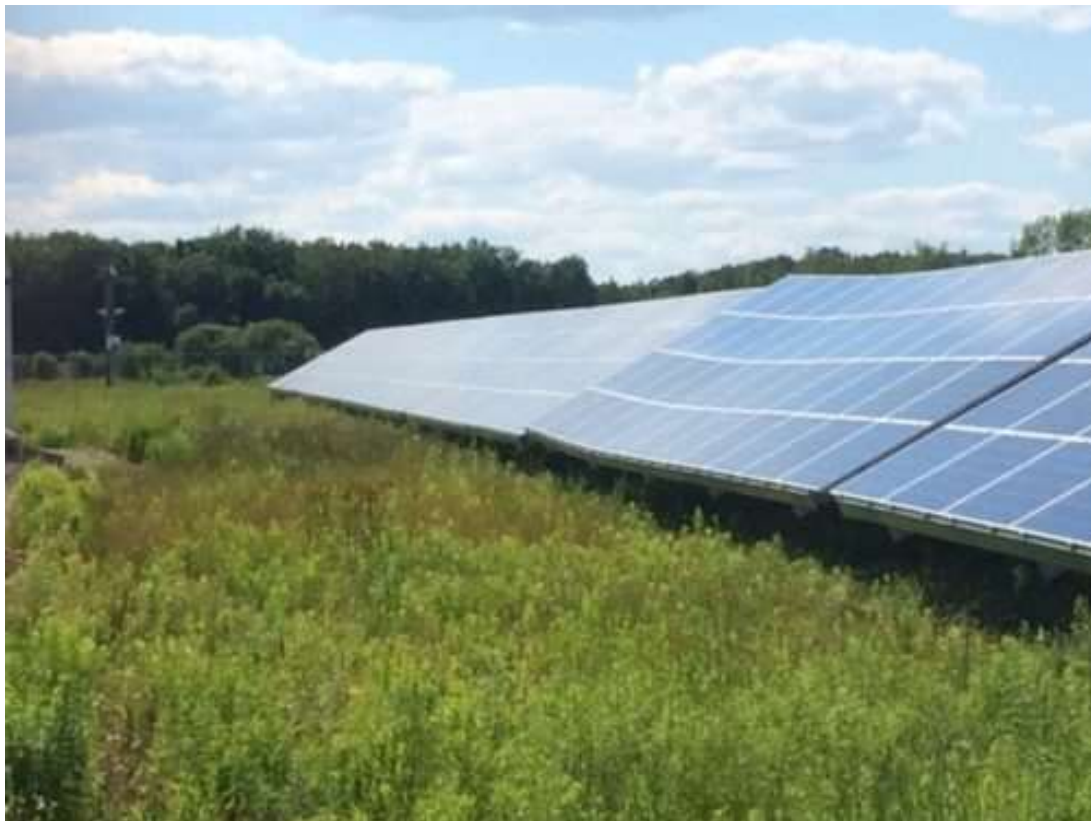
Figure 32 - Modules Mounting Structure sinking due to soil movement.
