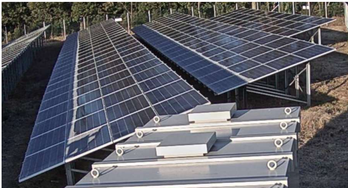
Figure 54 - Thin layer of ice over modules and row-to-row shading.
