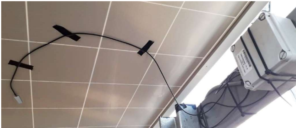
Figure 56 - Temperature sensor attached behind the module.
