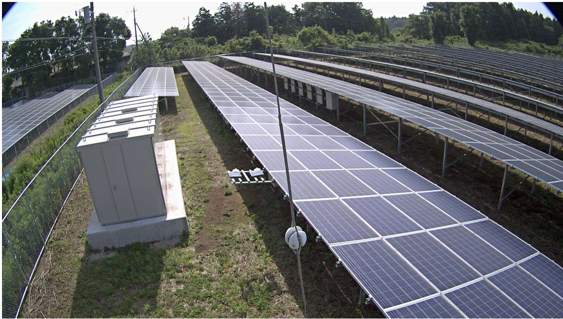
Figure 52 - Transformer station painted in white color creating false reading in the irradiance sensor.
