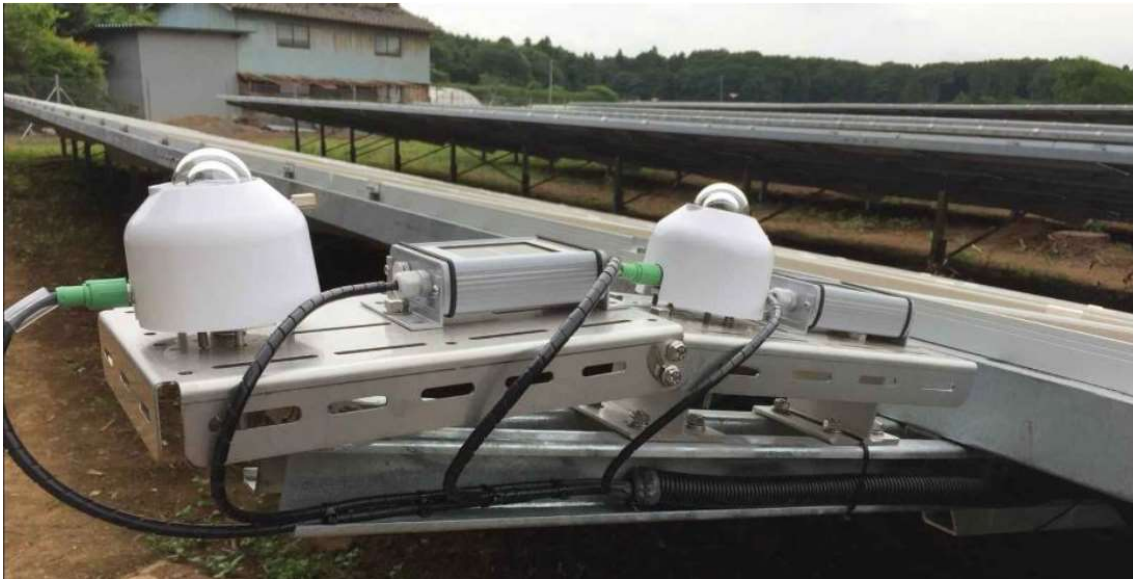
Figure 46 - From left to right: Horizontal Pyranometer, horizontal reference cell, tilted Pyranometer, tilted ref. cell.
