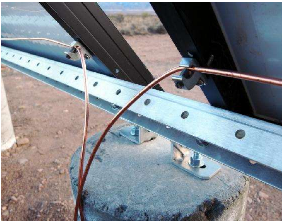
Figure 45 - Bare cooper wire for earth grounding.
