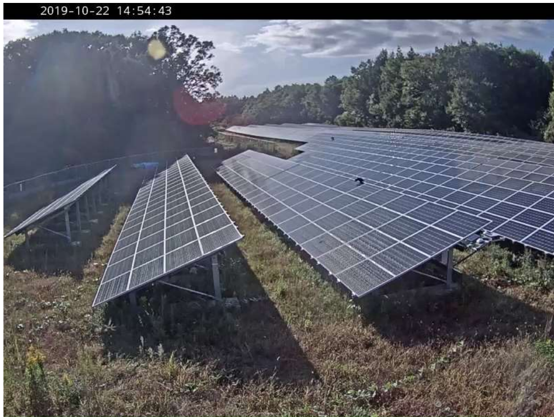
Figure 34 - Trees outside the power plant terrain causing shadow on the modules.
