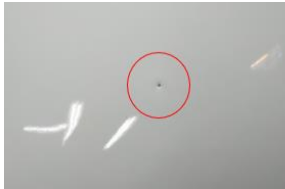
Figure 17 – Pinholes in sanitary ware
