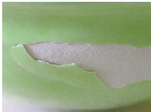
Figure 19 – Shivering/peeling in sanitary ware [49]
