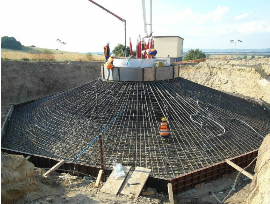
1. Complete reinforcement structure, formworks on both lower and upper part of the foundation.
