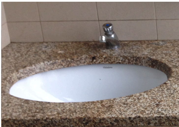
Figura 51 - Torneira instalada na IS
