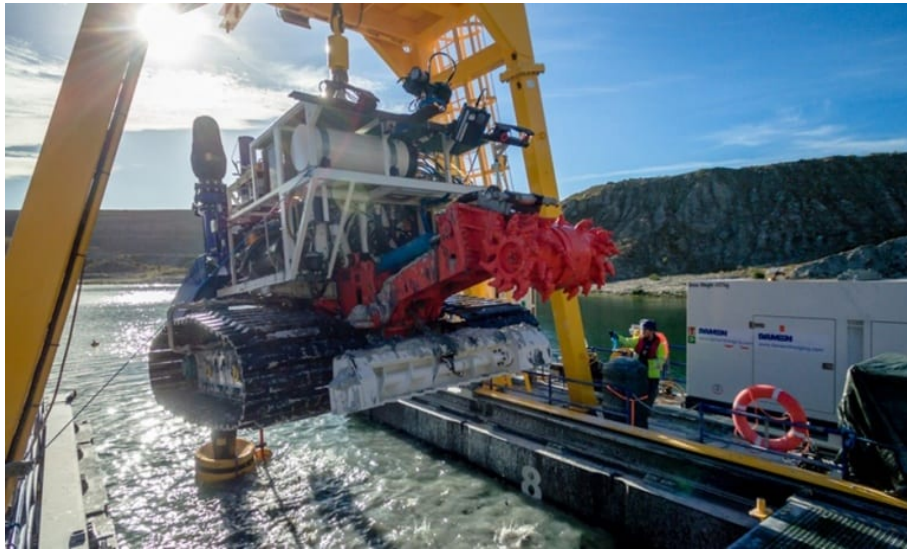
Figure 1.9: Mineration structure used in the VAMOS project
