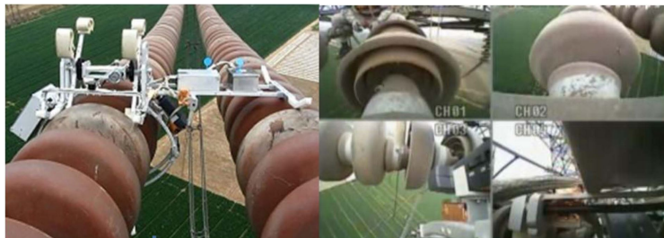
Figure 2.3: Insulator inspection robot. This robot has cameras installed for visual inspection and also perform electrical tests (Source: [29]).
